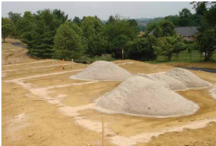
Tee construction underway at Lakewood Country Club in Rockville, Md. Among the elements key to successful tee work are proper subsurface drainage piping and tested and approved drainage gravel and tee soil mix.
