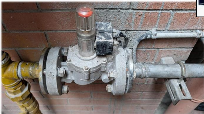
At first glance what was assumed to be a water valve is a gas pressure regulator.
