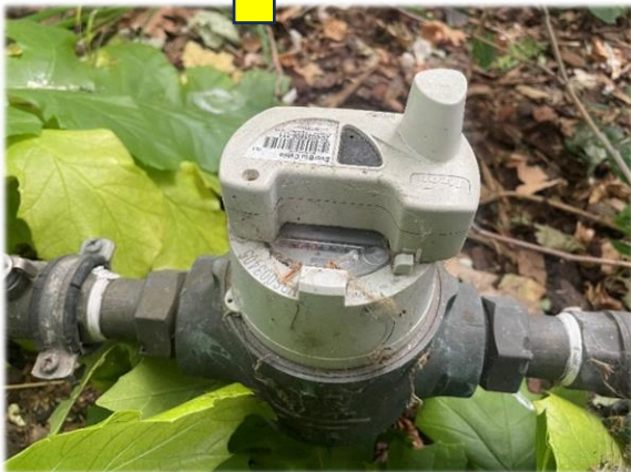
Installed is Itron TD8 25mm rotary piston PD Water Meter with Cyble AMR module.
