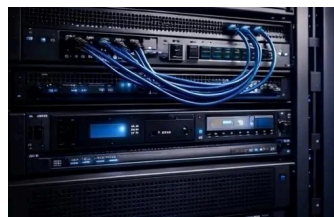
Network Rack & Low Voltage Installation
